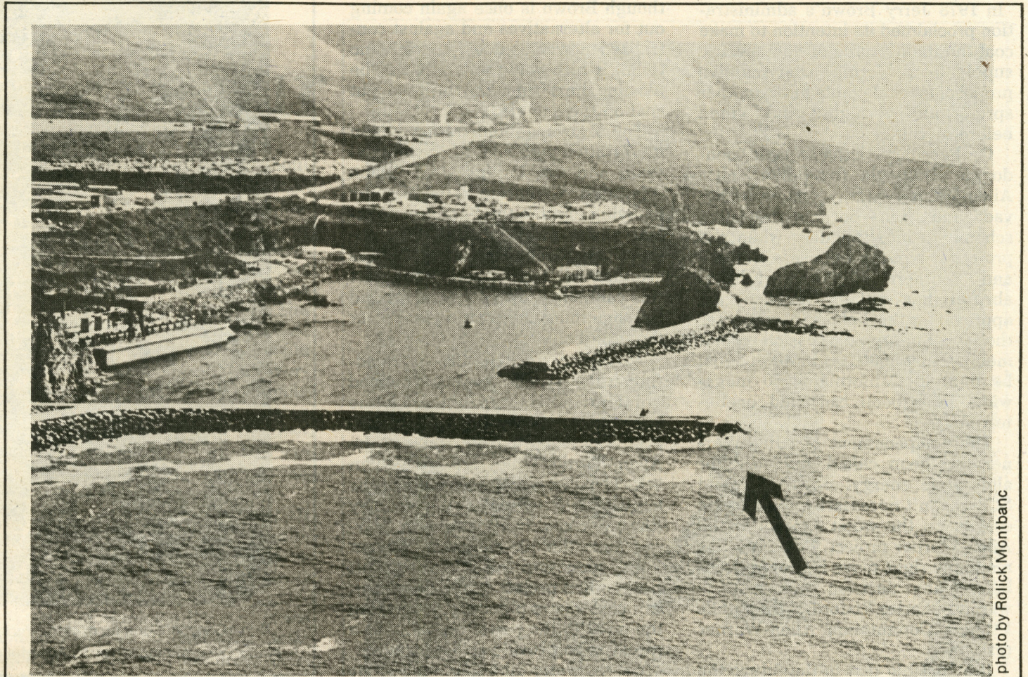
A quarter of the outer protective breakwater at the Diablo Canyon nuclear power plant was leveled by a seasonal storm.
